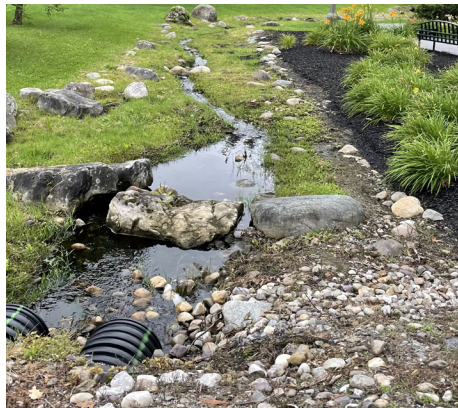
▲ Existing portion of stormwater management system
